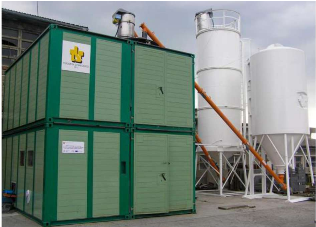
The production technology in the mobile version - the facility in operation
